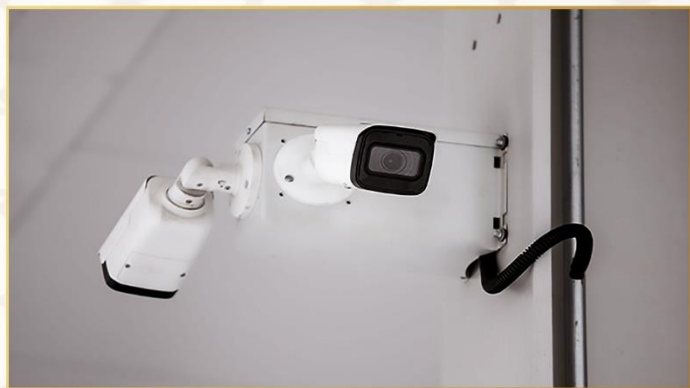
CCTV in Common Area
